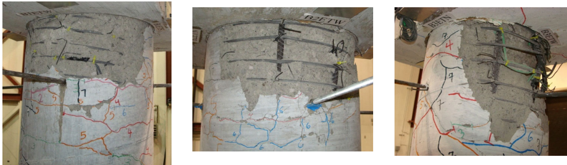
Fig. 7. Upper plastic hinge after final motion: left to right, SMA pier, PT pier, and ISO pier
