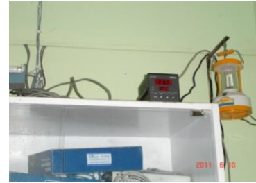
Fig. 11 Temperature data logger
