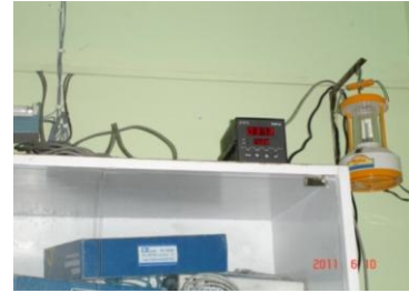
Fig. 11 Temperature data logger
