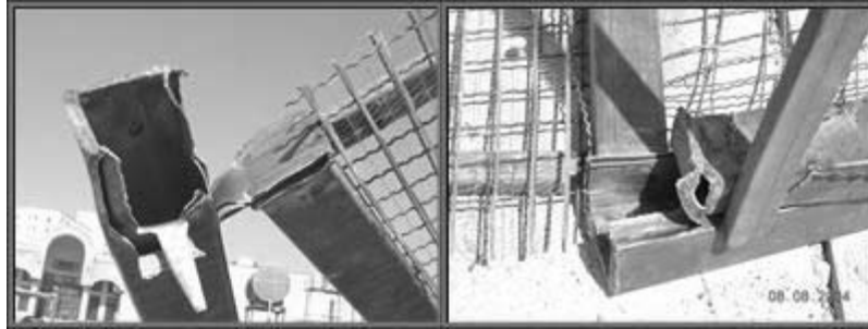
Fig.7 Destruction of beam to column moment connection
